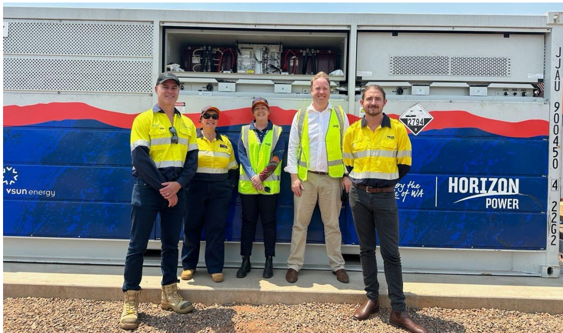
Figure 3 – Mr Zamien Sumich (VSUN Energy), the Hon David Michael MLA, Minister for Mines and Minister for Goldfields-Esperance, and Horizon Power’s team including Executive General Manager Jennie Milne, Alana Trew and Dylan Hearty at Horizon Power’s VFB BESS delivered by VSUN Energy
