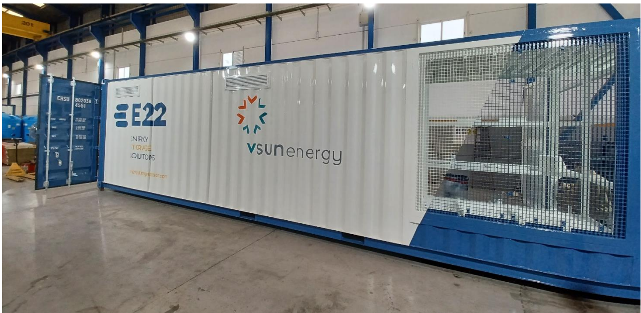
Figure 1 300kWh VRFB during construction at E22's facility in Spain
