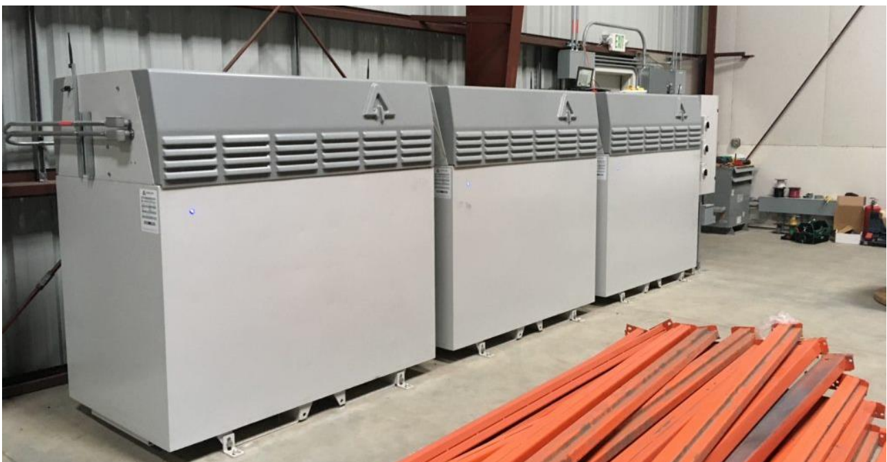
Figure 2 Avalon Battery VRFBs
