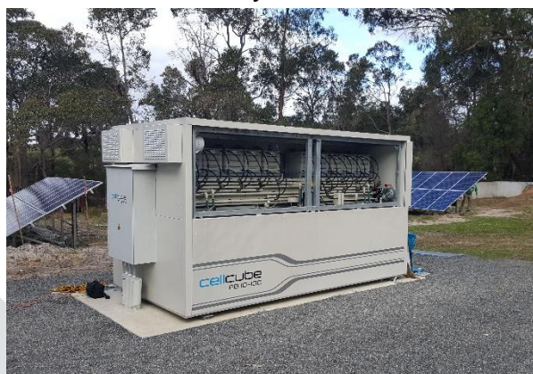
Figure 1 Vanadium redox flow battery in Busselton, Western Australia
