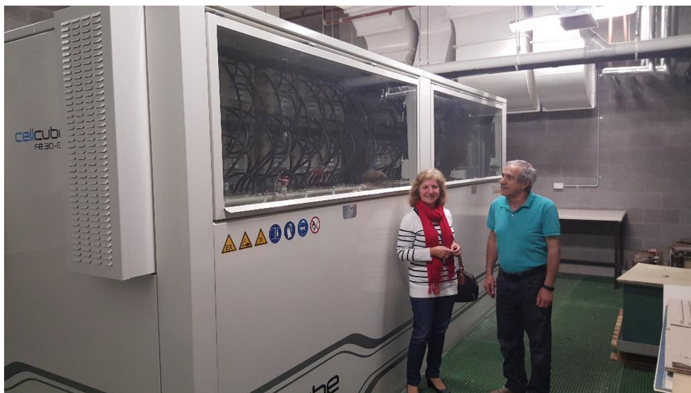
Fig 1. Emeritus Professor Maria Skyllas-Kazacos of the University of NSW and Michael Kazacos with the Vanadium Flow Battery installation at the UNSW
